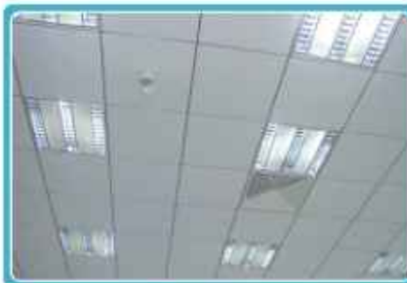
▶ Grid False Ceiling
